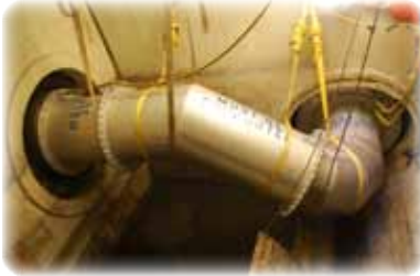
Flow Diversion in a structure. 48" pipe with a 24" bypass, flowing uphill.
